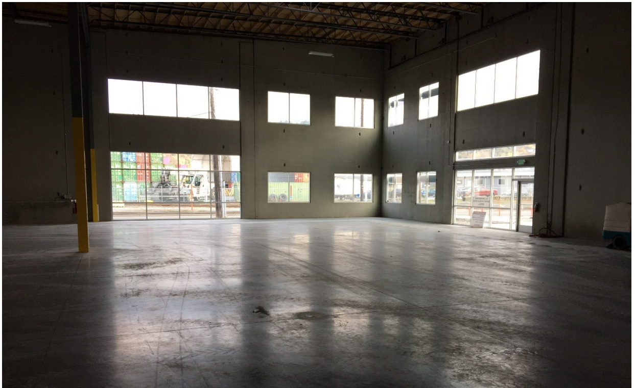
Photograph 12. NE Office Node of Building A. Passive Vapor Mitigation system located under slab.
