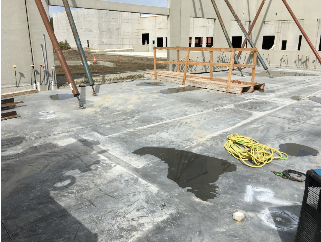
Vapor Pins VP-12 and VP-13 adjacent to northwest office in Building B in Ecology adjusted locations. Looking north-northwest
