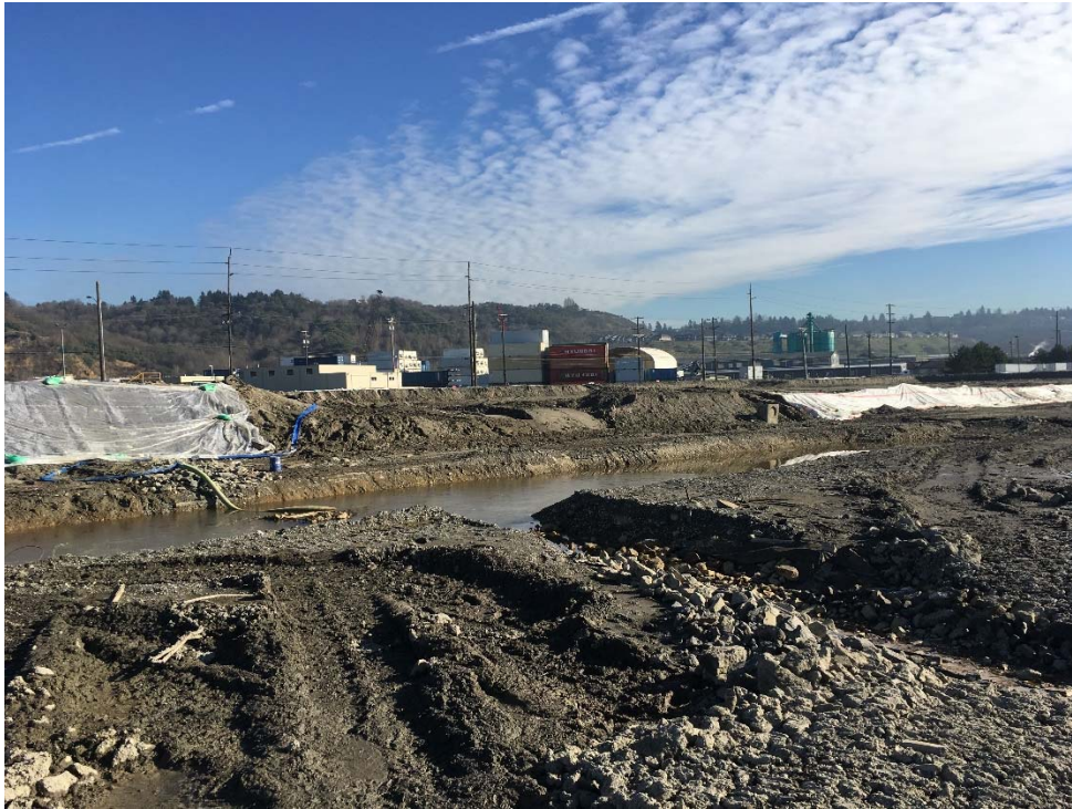
Caption: Standing water in stormwater pond (photo taken on site visit 2/13)
