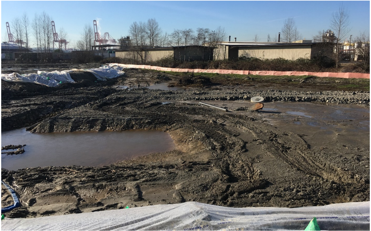
Photograph 7. Site conditions during second VOC vapor sampling event in May 2018.
