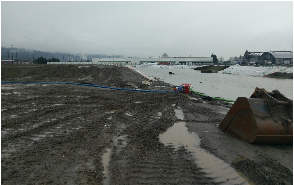
Photograph 6. Stormwater pump brought in to control excess water in the stormwater pond. Looking South
