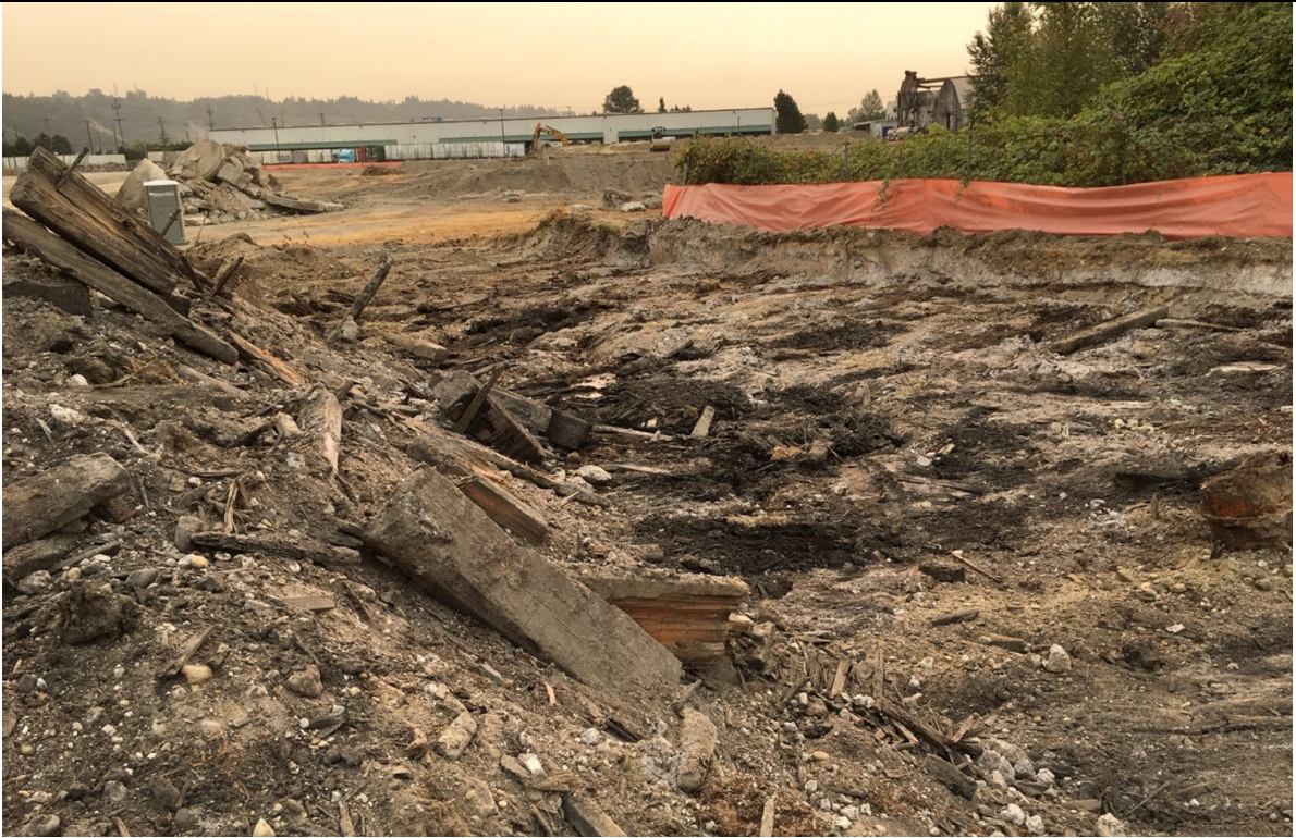
Photograph 3. Wood debris found in soil at the North west edge of property. Looking South
