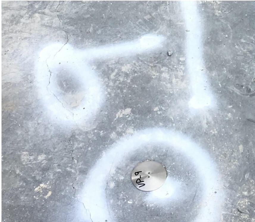
Photograph 4. Vapor pin with flushed-cover.
