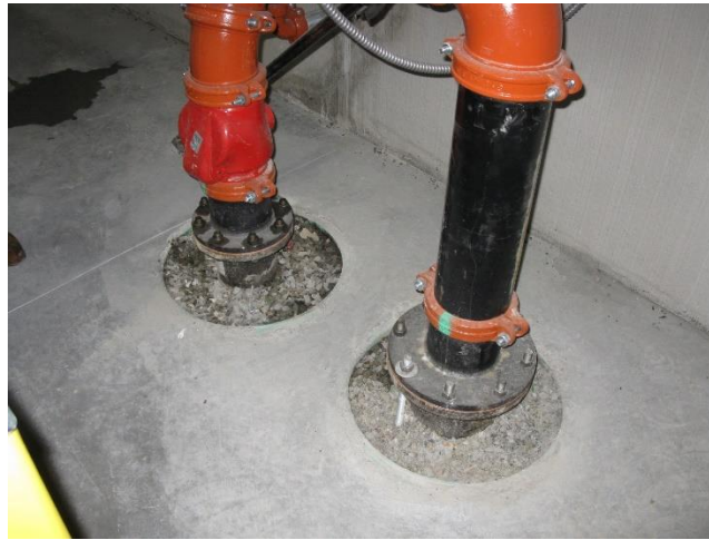
Figure 1. Note exposed gravel around fire supply water pipes that allow a direct connection to subsurface soil vapor.
