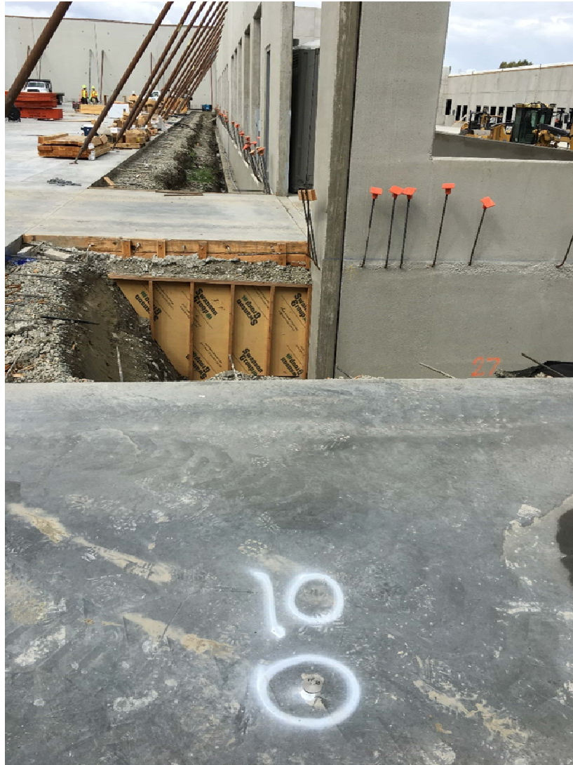
Vapor Pin VP-10 in Ecology adjusted location with stainless-steel cover. VP-10 is adjacent to the northeast office room in Building B. Looking west-northwest
