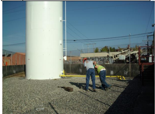
Photo #4: Secondary view of drilling at boring B-2, looking to the northwest. Note presence of the existing 30k gal fuel tank in background.
