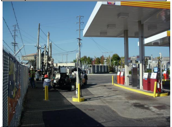
Photo #18: View of drilling at boring B-12, adjacent west of dispenser islands/associated underground storage tanks (looking north).
