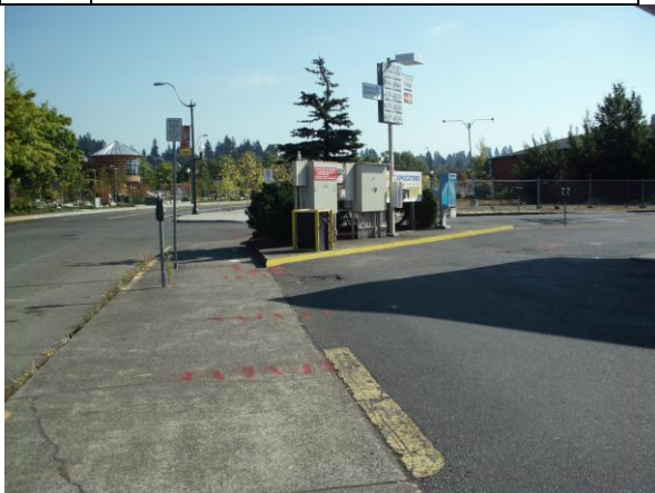
Photo #11: View of underground utilities markings adjacent north of Site on Thurston Ave NE sidewalk (looking to the northeast).
