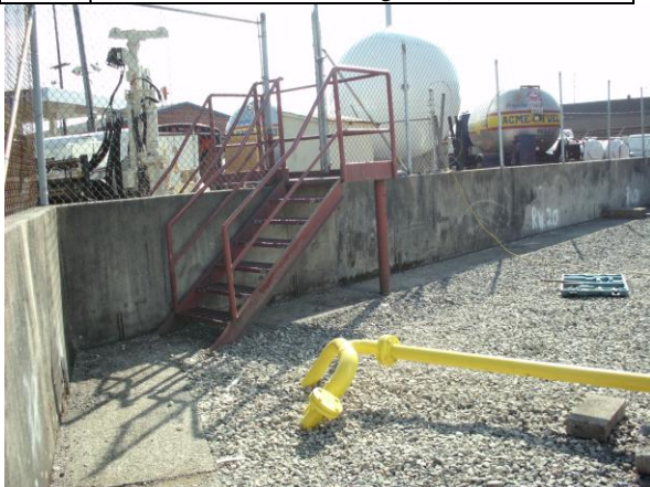
Photo #5: View of secondary containment area within the bulk fuel plant area at Acme (looking southeast).
