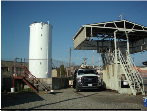
Photo #1: View of direct push probe drilling at boring B-1 adjacent north of bulk fuel area (looking northwest).
