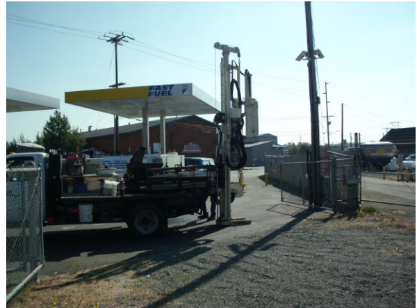
Photo #8: View of direct push probe drilling at boring B-6, east of bulk fuel tank/spill area on Cardlock facility area (refer to Figure 2).
