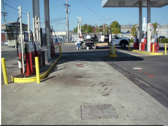
Photo #13: View of direct push probe drilling at boring B-8, north of dispenser islands and underground storage tanks at Cardlock facility (looking north)
