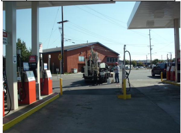
Photo #16: View of direct push probe drilling at boring B-10, adjacent south of 2 dispenser islands and associated underground storage tanks Looking southeast.
