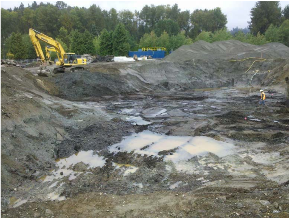
Photo 2 – Peat layer and water table exposed in southern extent of excavation (looking to south) on September 17, 2010.
