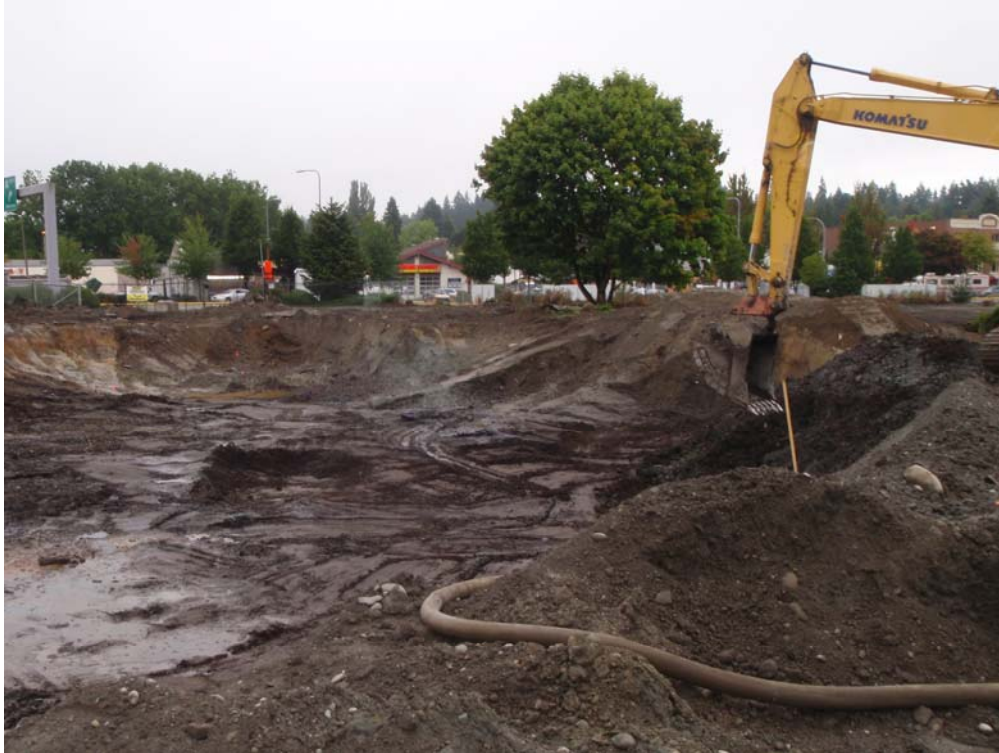
Photo 3 – Peat layer and water table exposed in northern extent of excavation (looking to north) on September 17, 2010.
