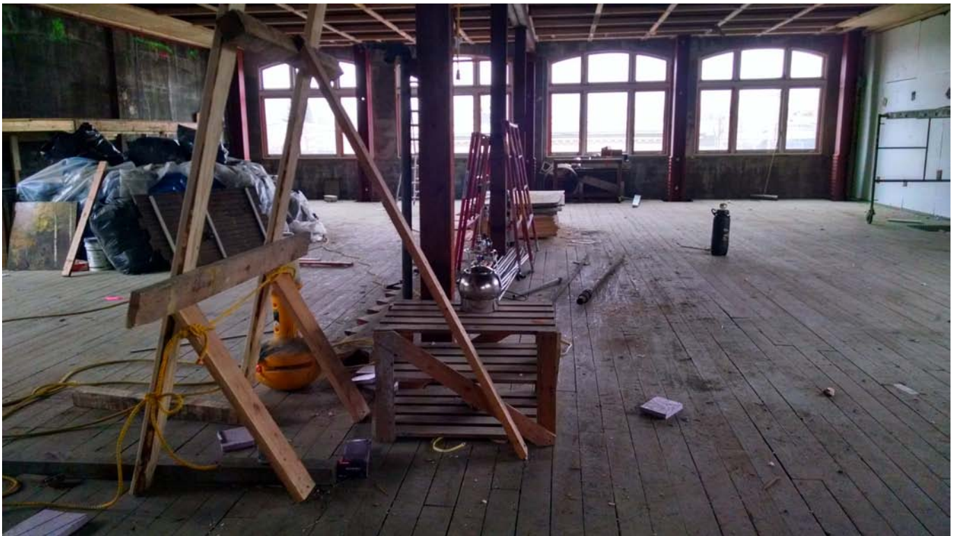
View of the indoor sampling location in the east end of the 2 nd story of the building, Jan 2018 (map ID#2)
