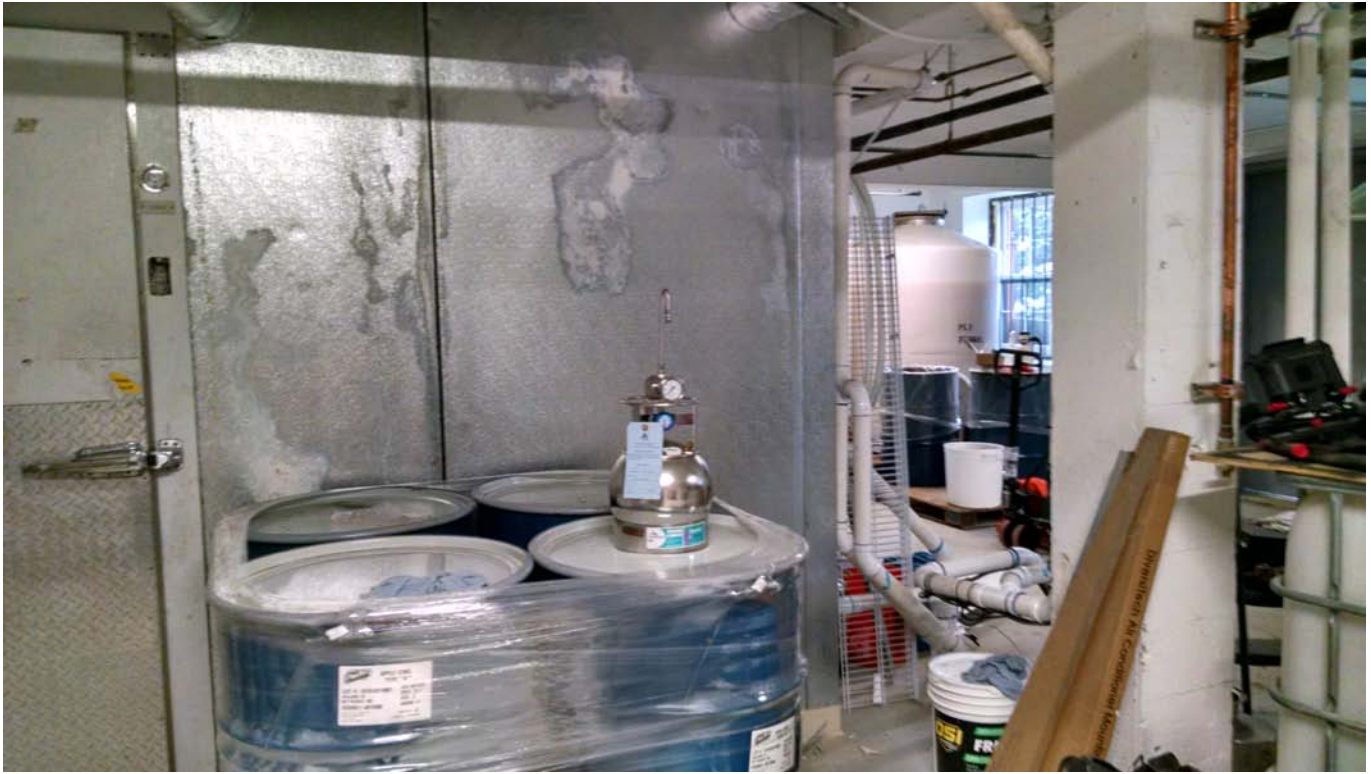
View of the indoor air sample location within the basement of the building, Jan 2018 (map ID#8). Sub-slab sample also collected from this location
