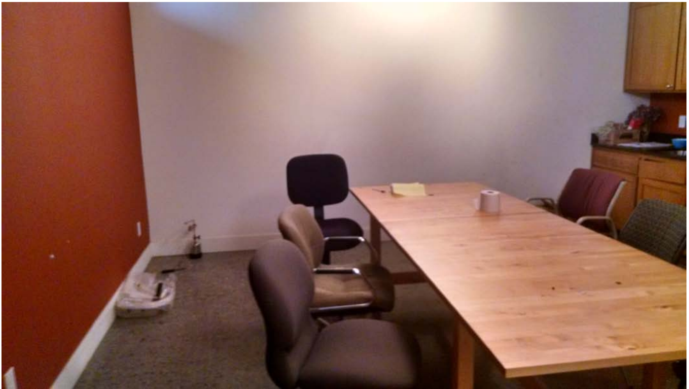
View of the sub-slab sample location within the conference room on the 1 st floor (map ID#6), Jan 2018. Indoor air and sub-slab sample collected from this location.
