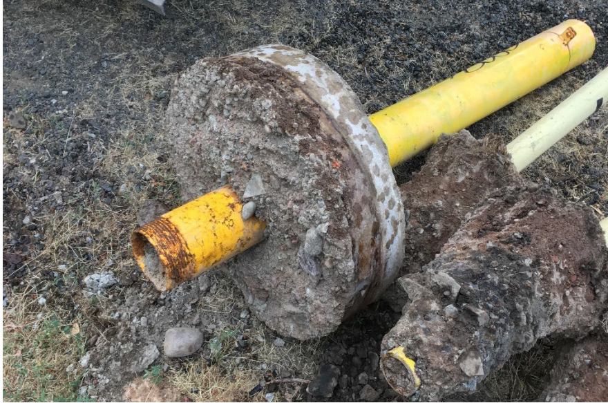
Figure 6: Well outer protective casing and monument removed for replacement with flush-mount monument. Requires a new measuring point (©2018, WA Dept. of Ecology).
