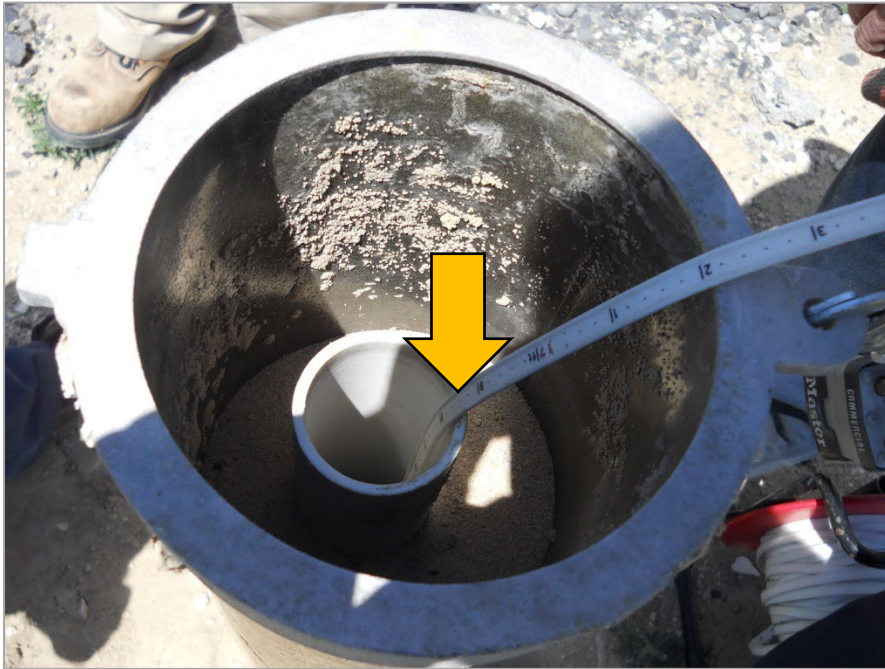
Figure 4: Arrow shows measuring point on a monitoring well, top of casing (©2012, WA Dept. of Ecology).
