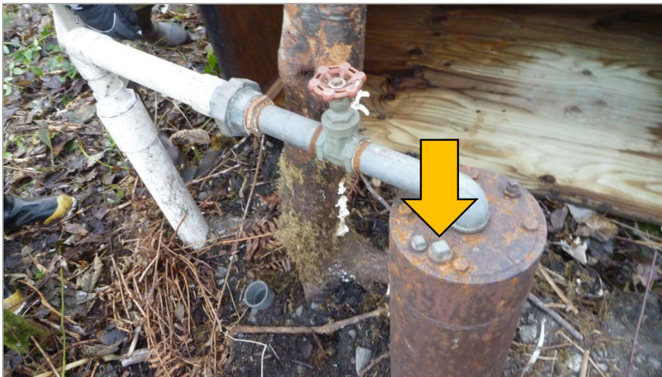
Figure 5: Arrow shows measuring point on a water supply well with access port (©2013, WA Dept. of Ecology).
