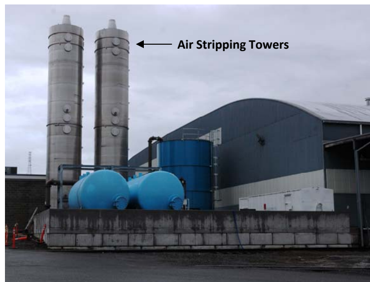
Groundwater pump and treat air stripping system.
