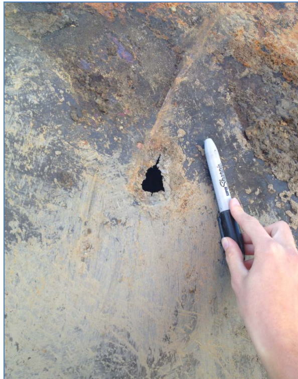
Hole in southern metal UST
