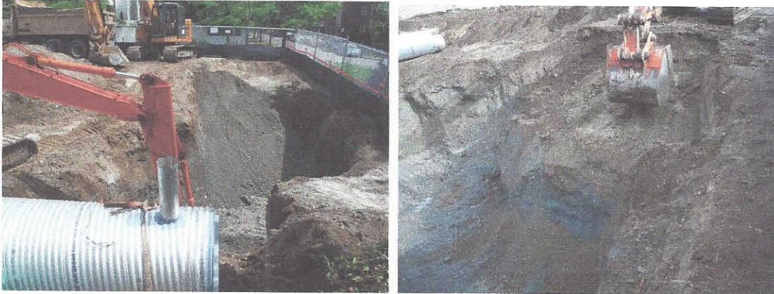
Photograph's above depict the ongoing excavation of petroleum contaminated soils at the site where clean overburden was removed from the upper layer and the grey/blue stained contaminated soils were removed and hauled away to a certified disposal facility as Petroleum Contaminated Soil (PCS),
