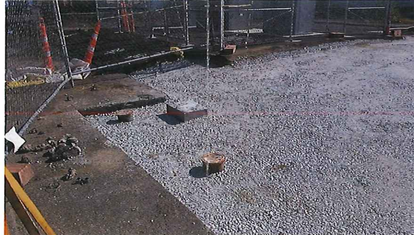
PHOTO 6 - LOOKING NE TOWARDS MWCP_104B, CP_104A, AND COMMUNICATION JUNCTION BOX
