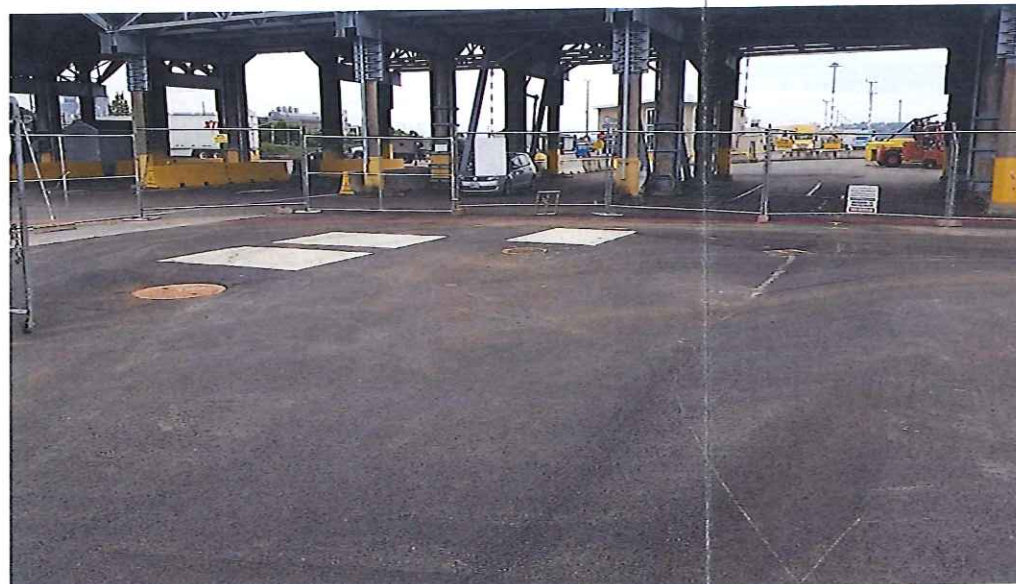
PHOTO 27 - LOOKING SOUTHEAST AT OIL WATER SEPARATOR AND WATER QUALITY VAULT
