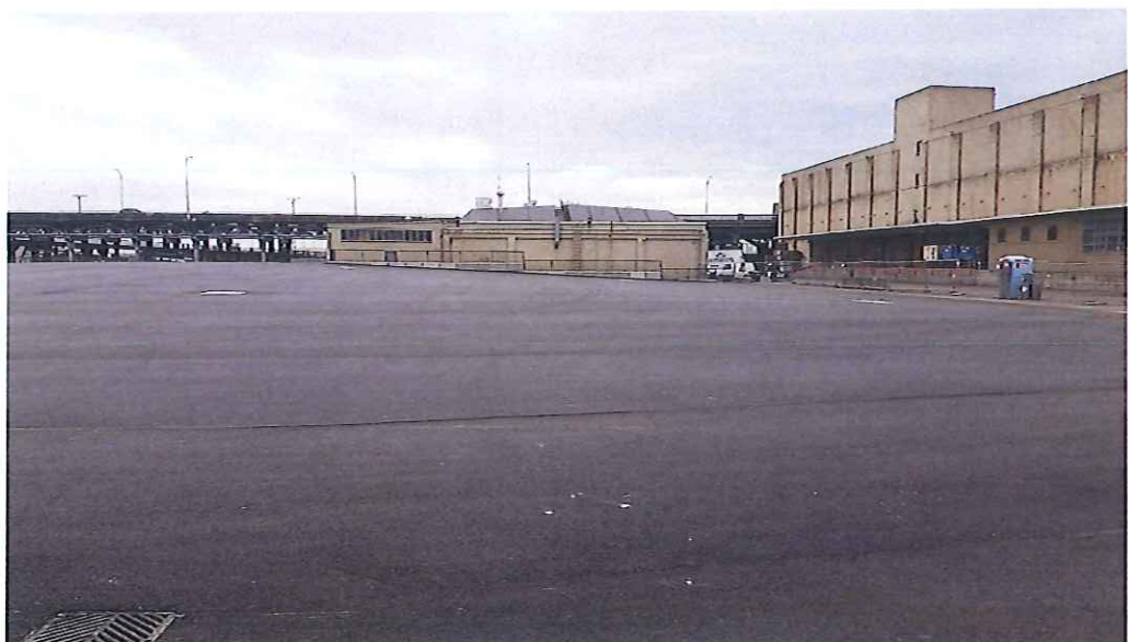
PHOTO 26 - FINAL ASPHALT COVER LOOKING SOUTH TOWARD BUILDING M-28. LNAPL TRENCH 3 VAULT LIDS VISIBLE MIDWAY FROM BUILDING M-28.
