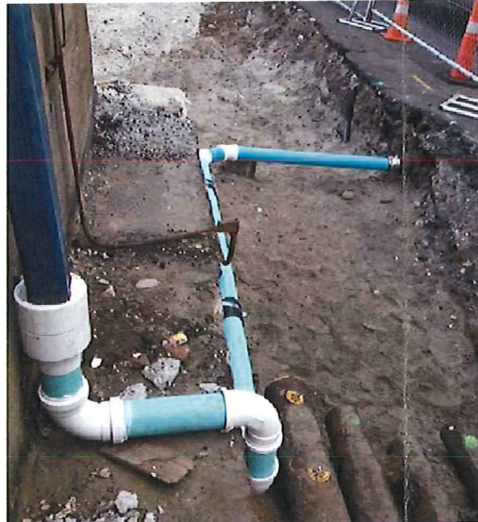
PHOTO 19 - LOOKING EAST AT THE NEW STORM CONNECTION ON THE SE CORNER OF BUILDING M-28
