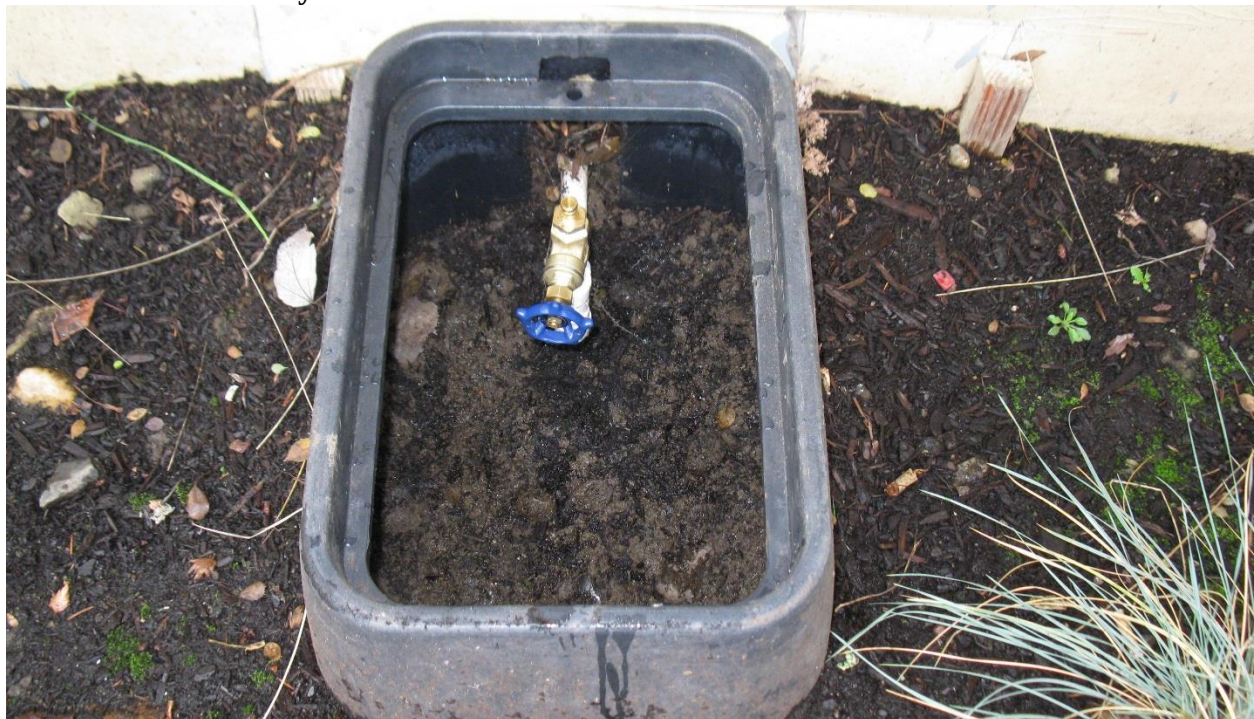
Photo 10: Soil Gas Vapor Monitoring Sampling Location/Port, Part of the Methane Mitigation System Installed between the Building Flooring and the Vapor Barrier Layer
