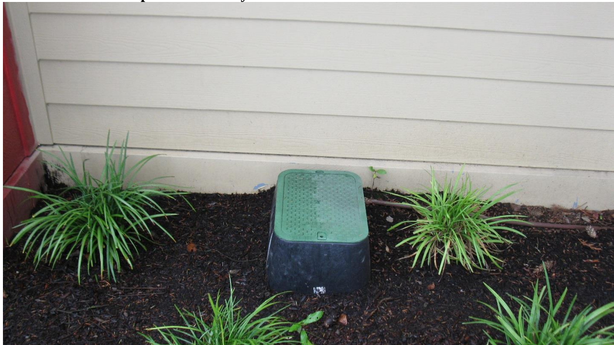
Photo 9: Soil Gas Vapor Monitoring Sampling Location/Port Box with the Top Cover, Part of the Methane Mitigation System Installed between the Building Flooring and the Vapor Barrier Layer
