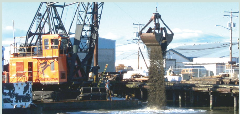
New, clean fill material being placed at site after excavation of contaminated sediments.
