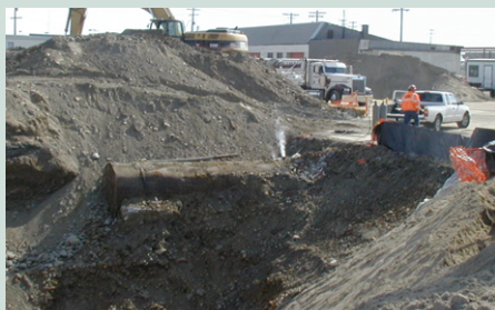
3,000 gallon underground storage tank being vented with nitrogen gas (photo courtesy of Dick Bassett)
