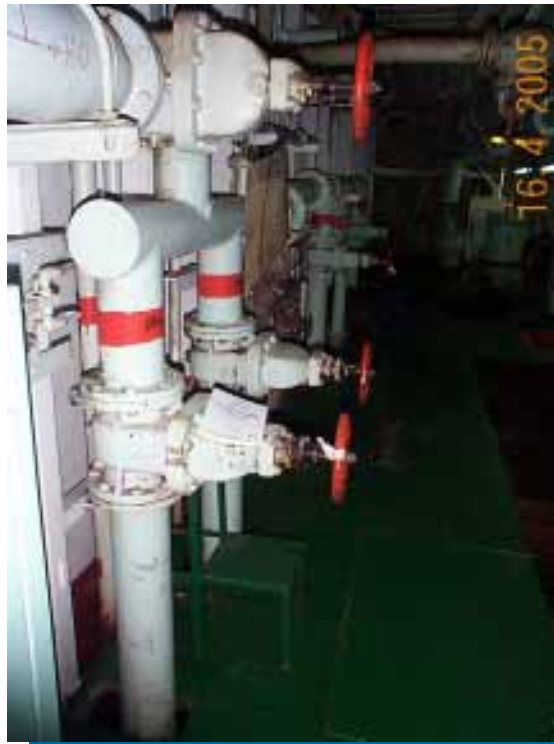
Figure 2. Fuel manifold at front bulkhead of the lower engine room of the PACIFIC EXPLORER [Note: The small piece of cloth tied to the valve handle was used to mark those valves being used during the transfer.]
