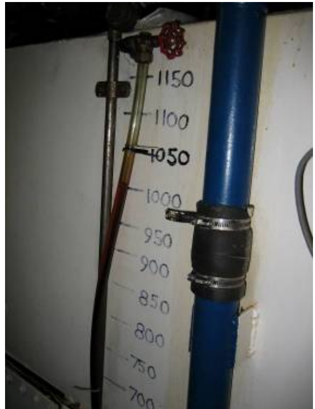
Figure 2 – Port day tank sight glass.
