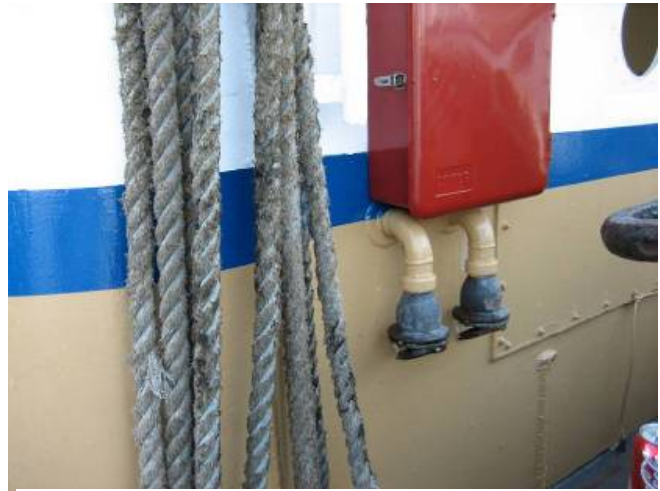
Figure 3 - Day tank vents located on the port side main deck of the CATHERINE QUIGG.
