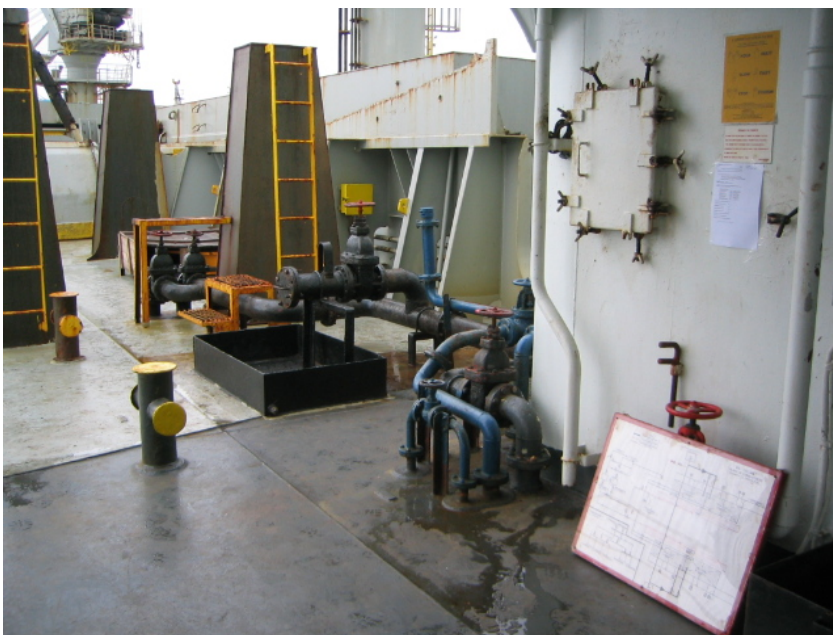
Figure 2 - Port side fueling station showing fuel oil header and tank drop line valves.
