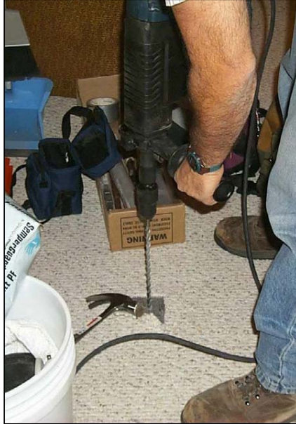
Figure D-1: Drilling through a concrete slab using a rotary hammer drill (Photo credit: EPA 2006)
