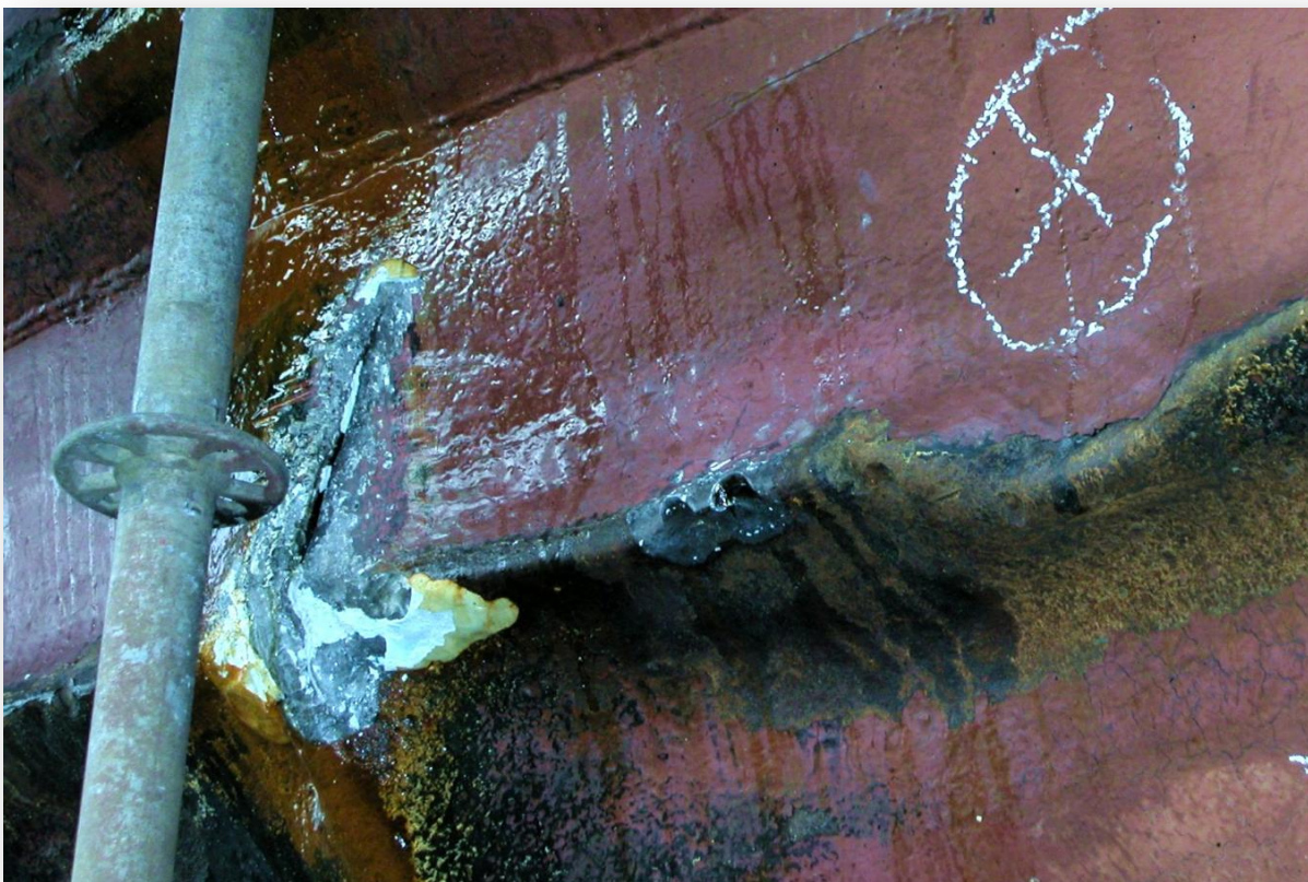
Damaged caused to the hull of a single-skinned tank barge as the result of hard contact between the tug and barge during berthing in rough weather. Oil leaked from the fracture upon loading the barge.
