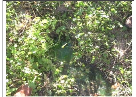
Dye pooling in the burrow-like hole formed at plugged outfall.
