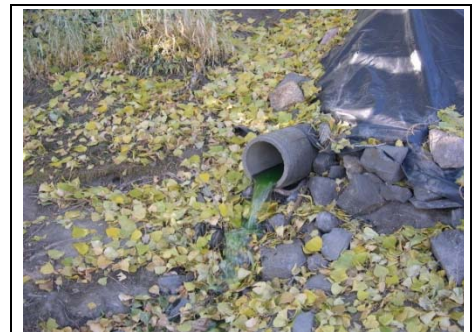
Dye test flow exiting one of the outfalls.
