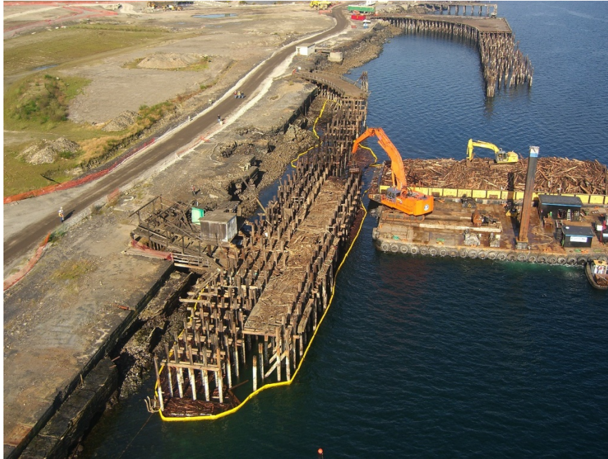
Figure 16-8. Removing pilings at the former Asarco Tacoma Smelter in Tacoma, WA. Boom is in place around the piling removal area and connected to a containment barge adjacent to the work platform.
