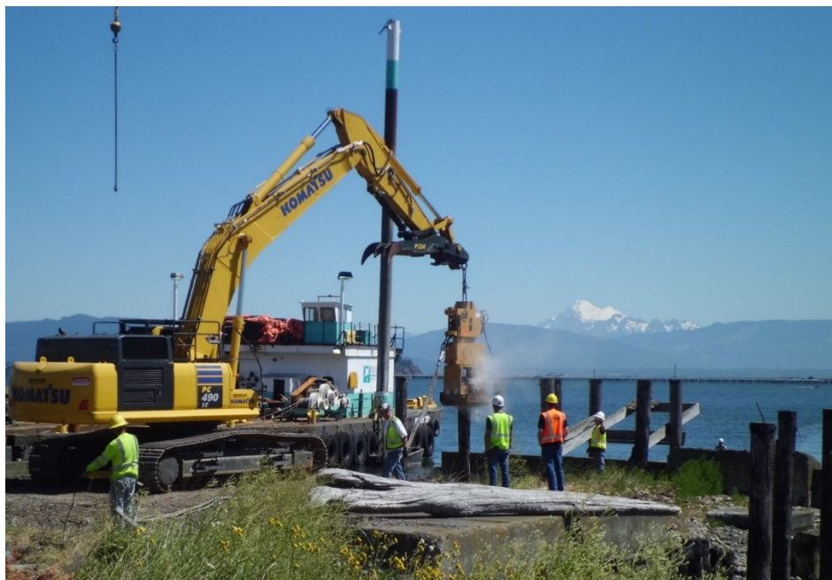
Figure 16-4. Piling removal using the vibratory hammer method. The equipment is parked on a concrete bulkhead at the former Custom Plywood mill site in Anacortes, WA. Some pilings took nearly 30 minutes to extract and produced smoke during extraction.
