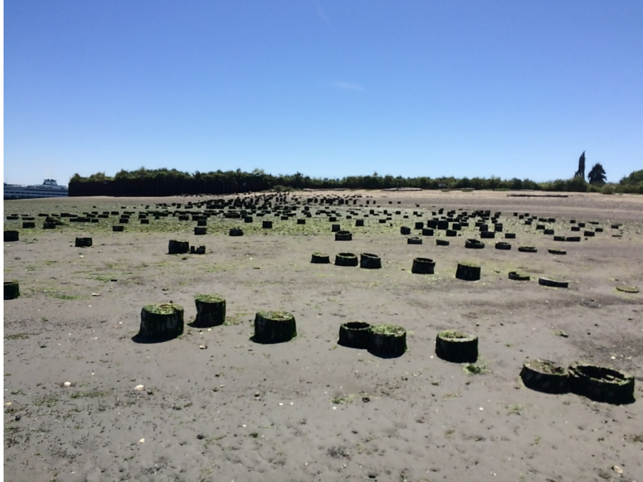
Figure 16-1. Cut piling stubs exposed on the intertidal beach at the Wyckoff Superfund Site on Bainbridge Island, WA. Pilings were cut at the mudline and wind and wave action exposed them over time.
