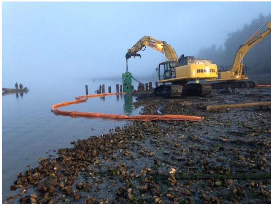
Figure 16-7. Removing pilings at the former mill site in Port Gamble Bay, WA. The boom around the piling removal area helps contain contaminants when the contractor is working the site during low tide.
