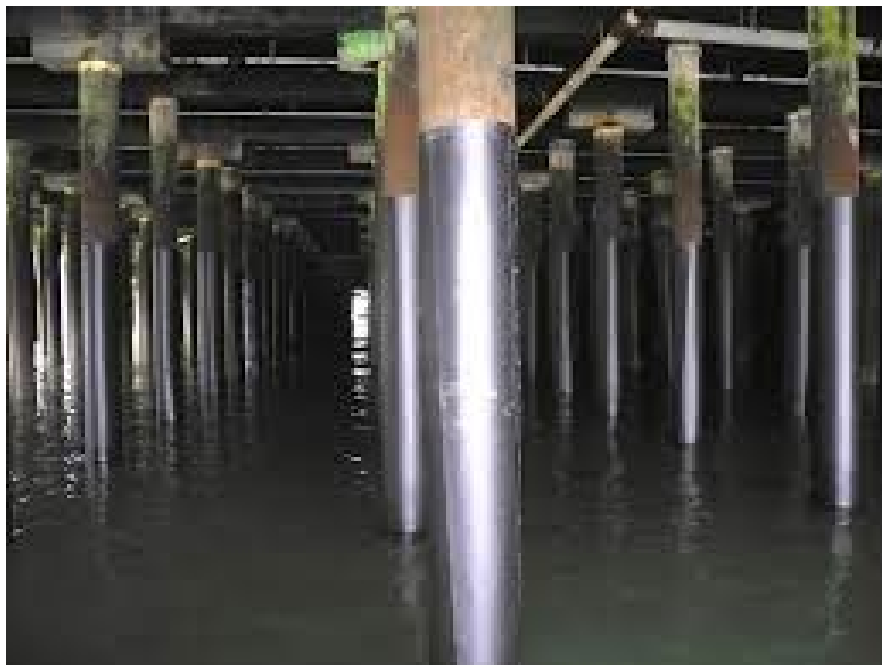
Figure 16-2. Wrapped piling at the Squamish Terminal in Squamish, British Columbia. Wrapped pilings protected spawned herring eggs attached to the pilings, which allowed the eggs to hatch.
