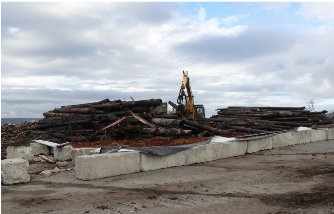
Figure 16-9. Piling removal containment area at the former mill site in Port Gamble Bay, WA. The containment area is constructed of ecology blocks, a synthetic liner, and wood mulch that prevent the release of sawdust, debris, splintered wood, and unfiltered water.
