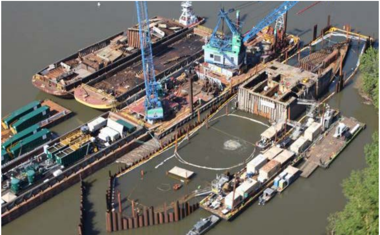
A coffer dam contained the Davy Crockett providing a safe work environment during vessel deconstruction.
