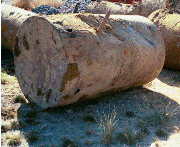
Figure 7.1 Removal of leaking underground storage tanks at Public Works facilities is a common use of Independent Remedial Action Grants.
