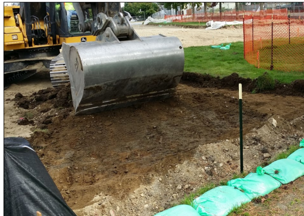
Contractors removed the top 12 inches of soil at Baltimore Park in Tacoma.
