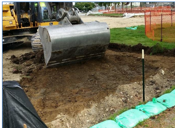
Photo 3: Contractors removed the top 12 inches of contaminated soil at Baltimore Park in Tacoma.
