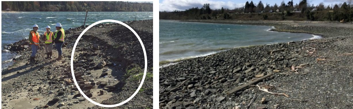
Figure 26 at left: Damage to the site after two severe storm events.
