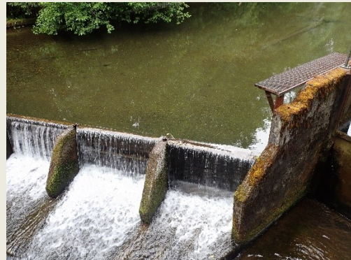
This structure on Bingham Creek has a fish ladder and smolt trap that have provided approximately 40 years of wild coho salmon life-cycle monitoring information.
