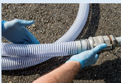
A hydrologist shows a long hose that delivers bacteria food to contaminated groundwater.
