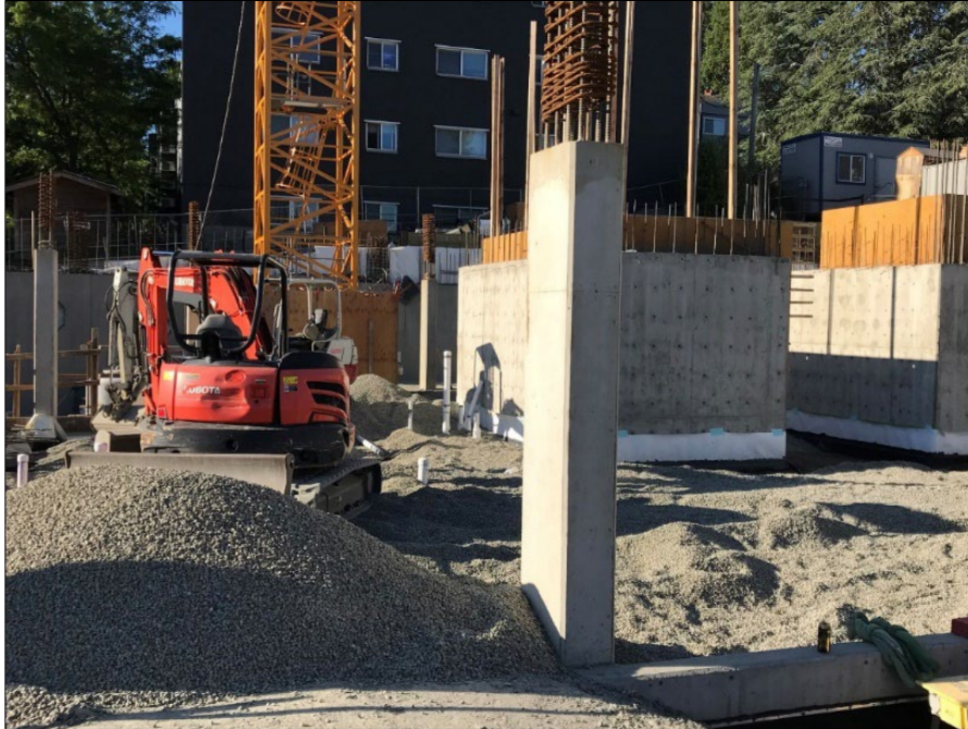
Figure 32: Construction is underway at the Mount Baker Properties Maddux Site after more than 13,000 tons of contaminated soil was removed. Ecology is partnering with Mount Baker Housing Authority to provide approximately 150 affordable housing units. Credit: K.Smith, Ecology (2021).
