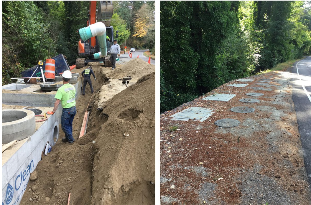
Figure 45: At left, workers install bypass piping between modular wetlands units on Marine Drive in the City of Bremerton, Kitsap County WA. At right, the newly installed underground modular wetlands units prevent roadway pollutants from harming salmon and shellfish beds in Oyster Bay in Kitsap County, WA. Credit: Ecology (2019)
