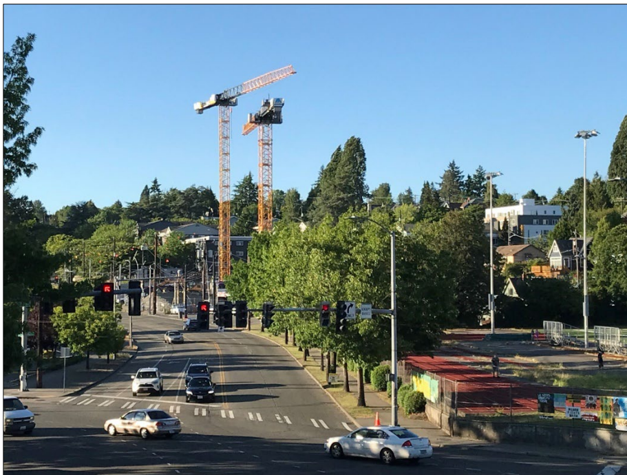
Figure 33: Two cranes tower over the Mount Baker Properties Maddux Site. The site is located in Seattle’s Rainier Valley neighborhood within easy walking distance of Franklin High School and the Mount Baker Light Rail Station. Credit: K. Smith, Ecology (2021).
