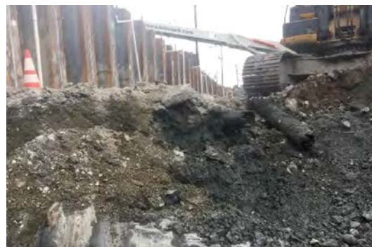
An abandoned heating oil tank.
