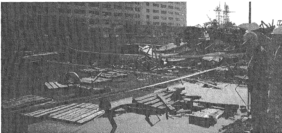
Military sites often contain contamination from past practices and are undergoing cleanup.
