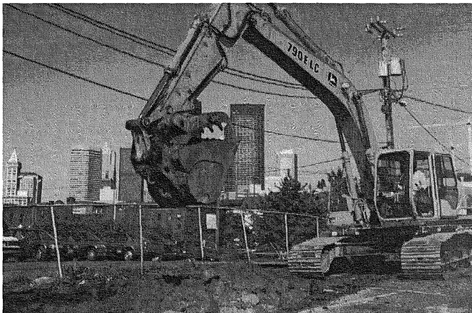
Bulldozer excavating petroleum contaminated soils at the Metro South Dearborn former bus fueling and maintenance facility in the Seattle Chinatown International District.
