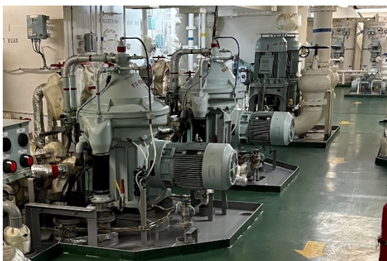
Fuel Oil Purifiers on a cargo vessel.
