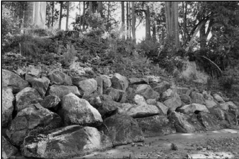
Figure 4. Riprap bulkhead/revetment located on northern end of Dick property and neighboring property.
