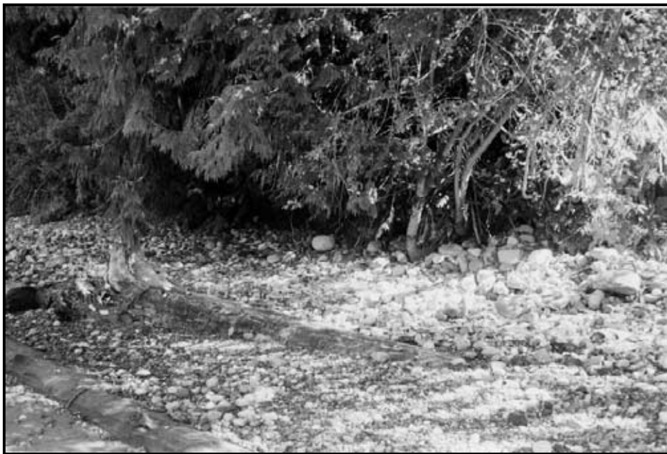
Figure 2. The toe of the bank had been undercut prior to construction. Quarry spall was placed in undercut area and logs anchored into the beach. Anchor cables are just visible.
