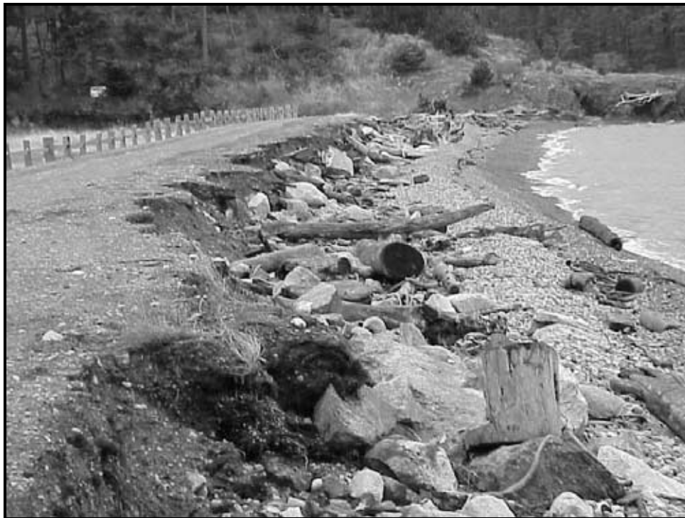
Figure 5. View north of project area prior to construction, showing erosional scarp in old fill, damage to road, and riprap ( Photo: provided by Jim Johannessen, Coastal Geologic Services, and Blakely Island Maintenance Commission ).
