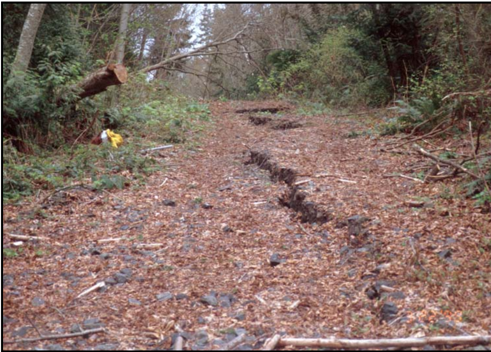
Figure 34. Fissure running down the center of the western portion of Ricky Beach Road. The shoreline is located over 100 feet to the right of this photo. [Photo: 3/22/1999, #99-12-8]
