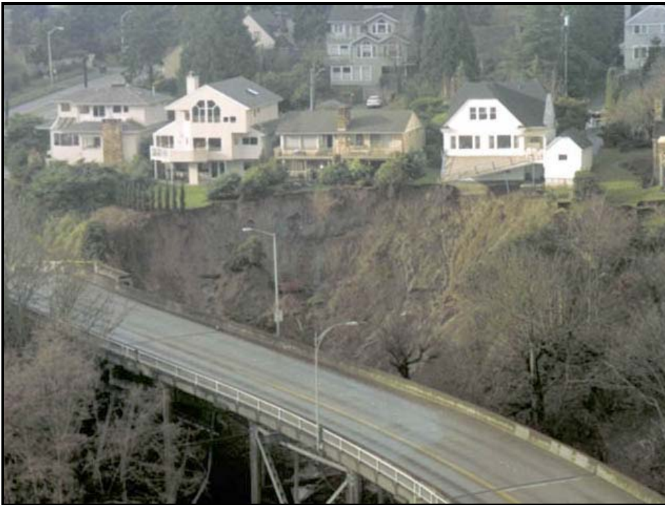
Figure 17. Landslide above Magnolia Bridge. In addition to threatening homes at top of slope, slide debris damaged bridge supports and a home located at the base of the slope. [Photo: 1/2/1997, #4108_14]
