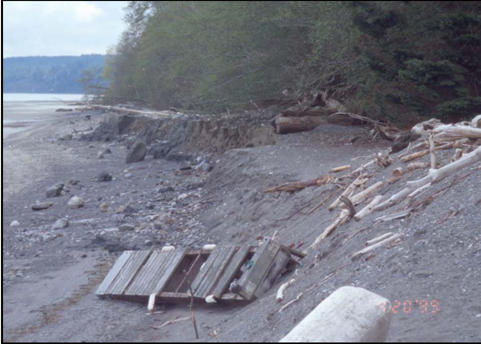
Figure 30. Toe of Thorndyke Road landslide, showing steep scarp has developed in the upper beach. [Photo: 4/20/1999, #99-21-22]
