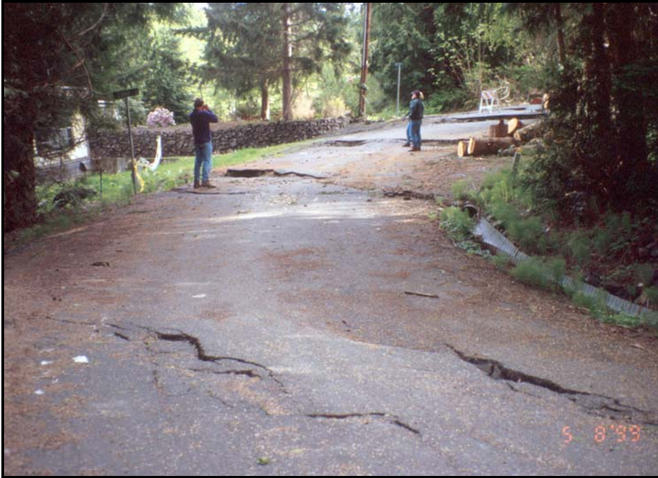
Figure 39. Fractures along Mariner Drive in eastern portion of Carlyon Beach neighborhood. [Photo: 5/8/1999, #99-25-14]
