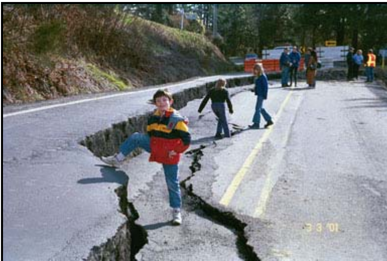
Figure 45. Reactivation of landslide along Highway 302 near Victor in Mason County. Field assistant is approximately 4.2 feet high [Photo: 3/3/2001].
