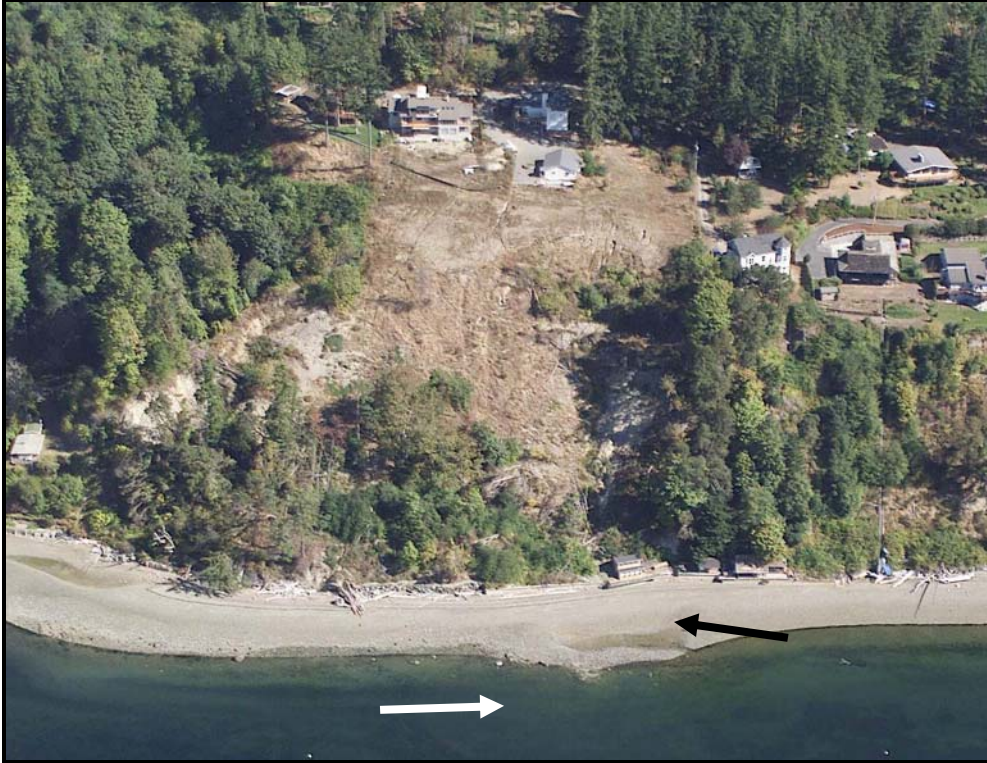
Figure 36. Aerial view of landslide south of Kamus Road on Fox Island. Photo was taken in summer, 2000, about a year and a half after the slide. Note how toe of slide affects shape of the beach. Arrows indicate locations of Figure 37 and Figure 38. [ Ecology, Kamus_2000 ]
