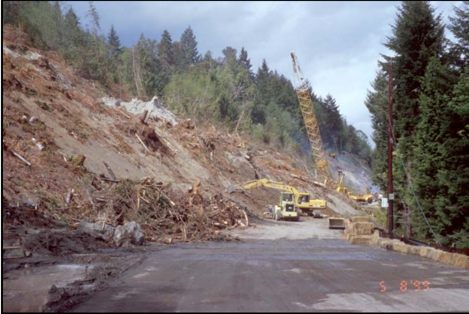
Figure 28. Highway crews attempting to clear highway and stabilize toe of Milepost 322 landslide. [Photo: 5/8/1999, #99-25-7]
