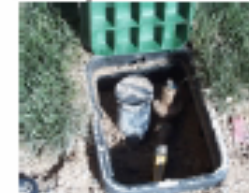
Sanitary Sewer "Clean Out"
