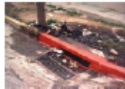
Dirty Storm Drain
