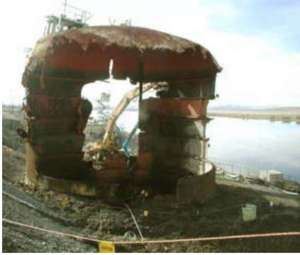
An old tank next to the Columbia River is torn down and will be safely disposed
