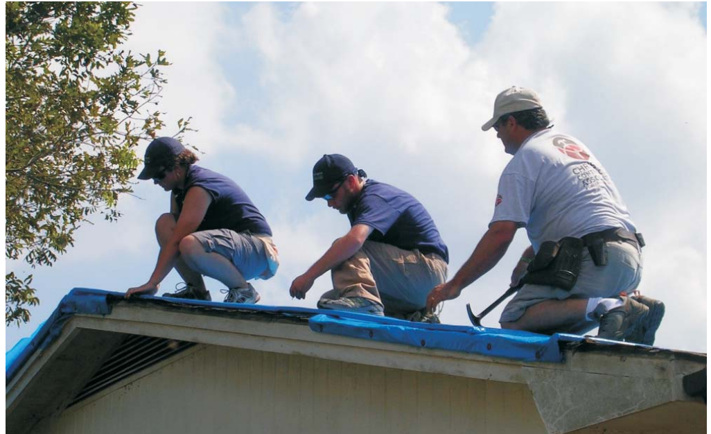
WCC members Vanessa Lott and Will Simpson work along side Scott Jager from the Christian Contractor's Association
