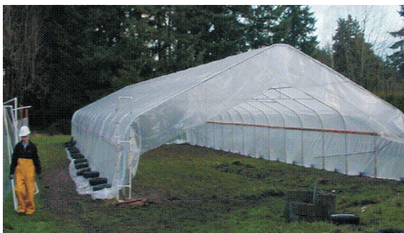
Greenhouse built by the Olympia spike crew (sup Dewees) and 5 Individual Placements for the non-profit Group, Garden Raised Bounty (GRUB)
