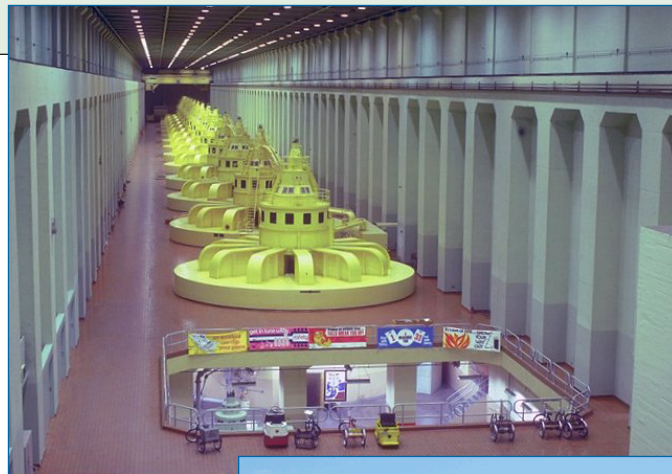
Turbines at McNary Dam on the Columbia River. Water passing through hydropower dams creates energy worth more than $3 billion per year.
