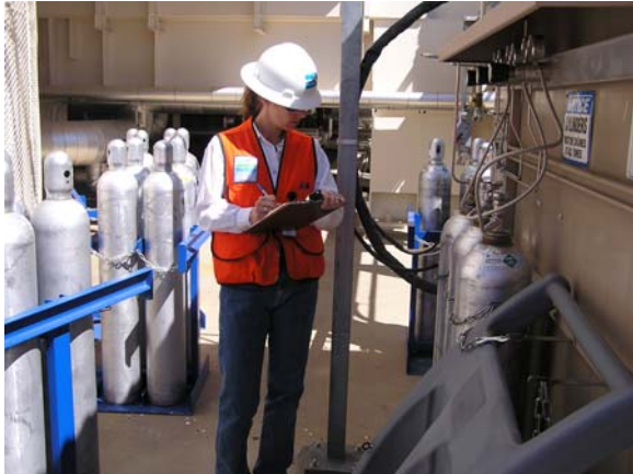
Lynnette Haller, air quality engineer, inspecting calibration gas canisters for a continuous emissions monitoring system.
