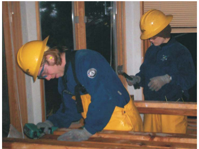
Crew Members Paul Griffith and Laila Murfin use a prybar and denailer to remove nails from salvaged lumber
