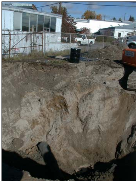
Picture showing excavation of contaminated soils at localized pocket at monitoring well (MW-8) October, 2003
