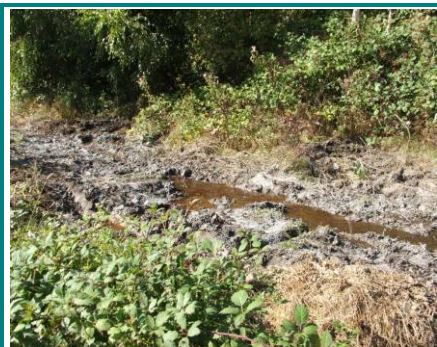
Freeland Plaza drainfield failure April 2006
