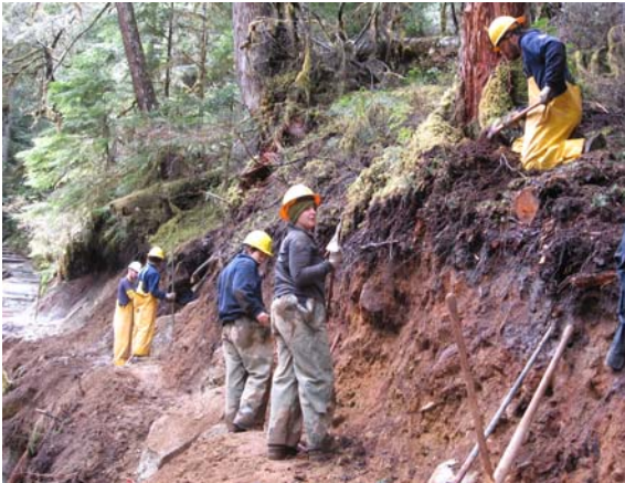
Olympia-based WCC Crew rebuilds trails that were washed out during the November 2006 floods near the Carbon River at Mount Rainier. From L to R: Ted Dewees (supervisor), Paul Griffith, Samantha Harvell, Tricia Bays, and Samuel Lanz.
