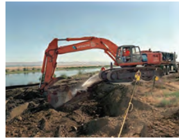
Soil removal is ongoing sitewide as a way to prevent contamination from spreading.
