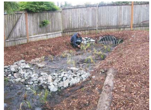
Ricky Porter plants sedges in the rain garden. A rock dam with curvature helps slow the water.
