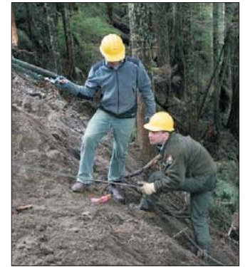
National Park service ranger and a WCC Corpsmember work on trail repairs east of Cougar Rock.
