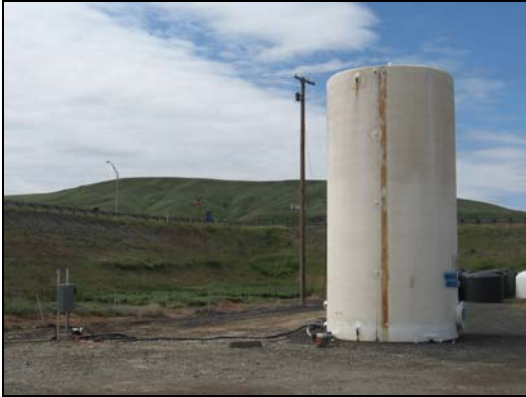
New brine storage tank
