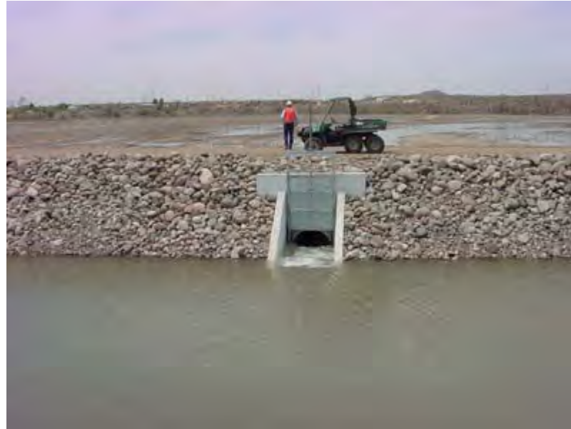
Operator Adjusting Gate at Basin Inlet Structure
