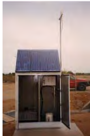
Solar Powered Remote Data Acquisition Site
