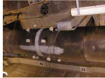
Typical Acoustic Flowmeter in Use at Pilot Facility
