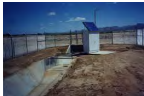
Solar Powered Remote Data Acquisition Station
