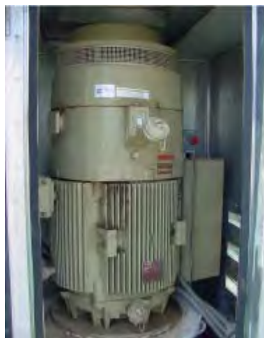
Electric pump at the HMRP turnout
