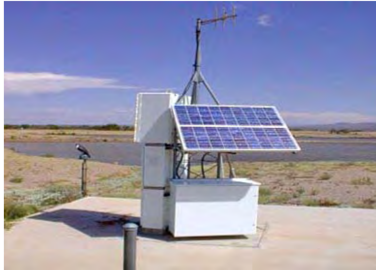
Solar powered remote data acquisition system at AVRP
