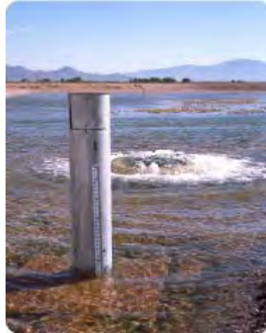
Stilling Well in the Basin With a Pressure Transducer Installed Inside (Basin 1)
