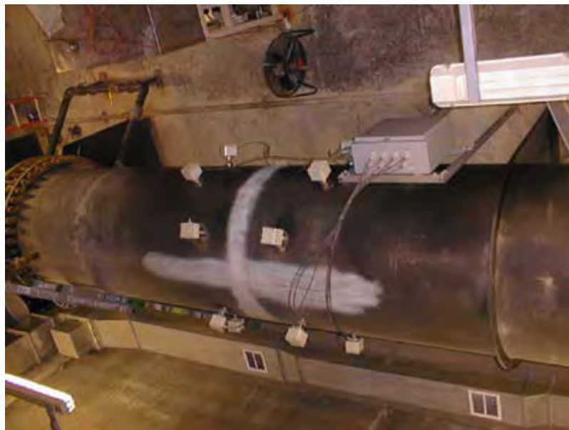
Acoustic Flowmeter at Blowoff Structure
