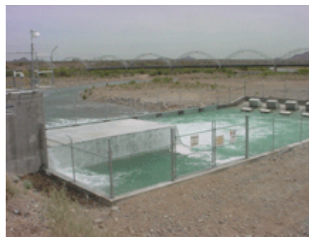
Blowoff Structure Releasing Water into the Agua Fria River
