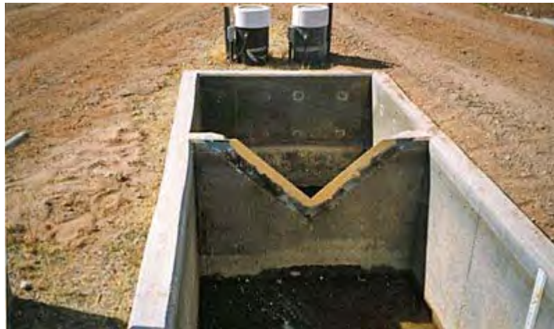
V-notch weir with stilling wells at top of photograph
