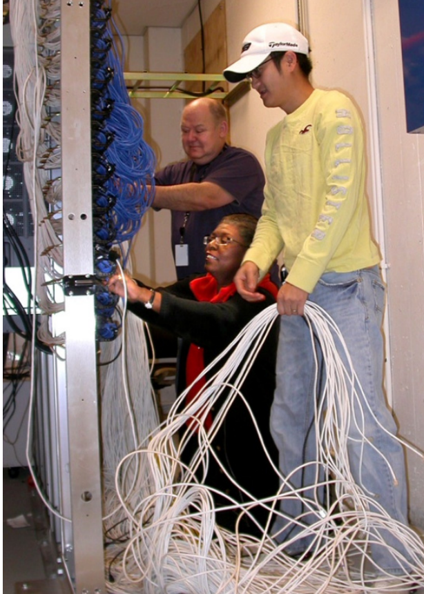
Ecology employees (from left) David Hovik, Gwen Campbell, and Shawn Lee work together on a network infrastructure upgrade project replacing cables in a communication closet at Lacey headquarters.
