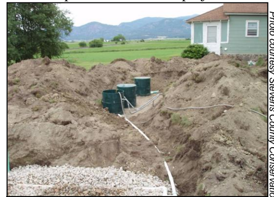
Septic tank and pump chamber
