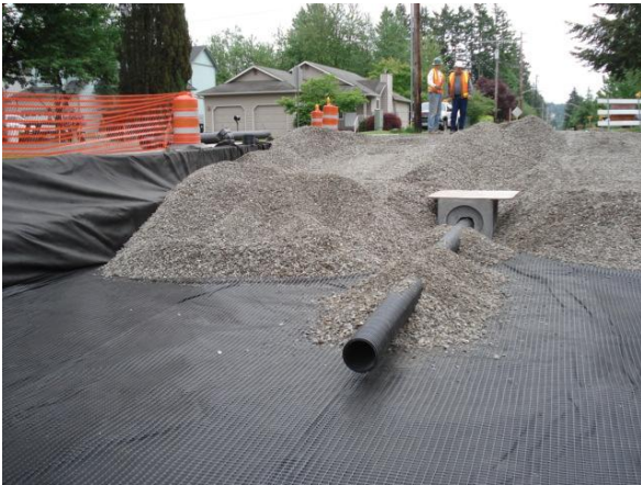
Underdrain system on impervious pavement. By Craig Tosomeen.
