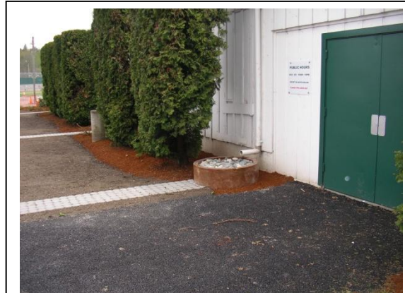
Porous asphalt walkway, Ecostone pavers, and compost amended soils in lawn and landscaped area.
