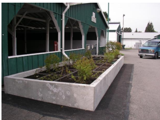
Biofiltration planter box installed to infiltrate roof runoff.
