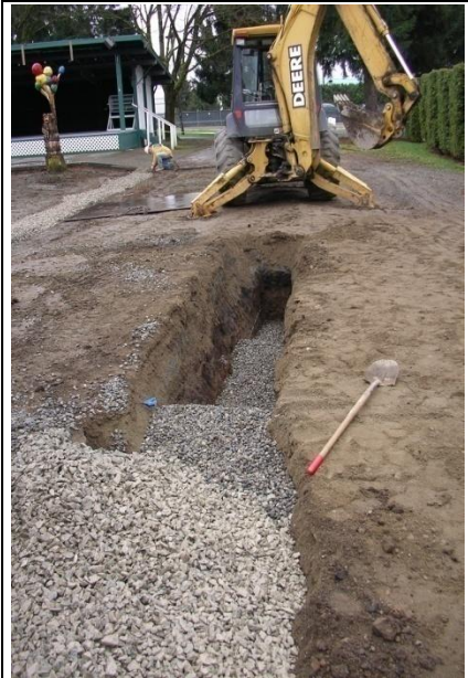
Infiltration trench installed to help runoff drain down to faster draining soils.
